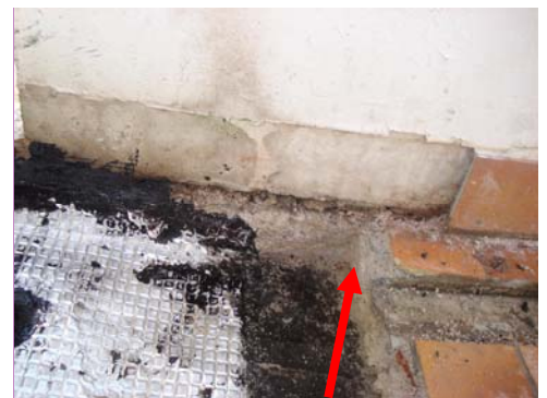
Terrasse MOMBELLI - Absence de joint
